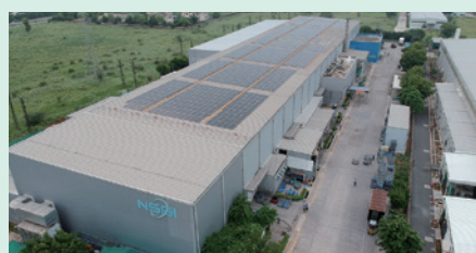
Roof-mounted solar power generating system at Neemrana Steel Service Center India Pvt. Ltd
